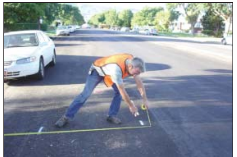
Lonnie Wolff of the Color Country Cycling Club assisting the Cedar City Engineering Office with marking of streets prior to the painting of bicycle lanes.
